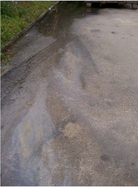
Figure 7: Sheen on parking lot
