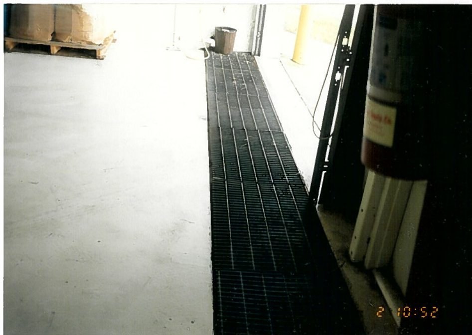
Photo 8b. Trench located in front of the Western doors within the Accumulation Center Drum Storage Area (SWMU 8).
