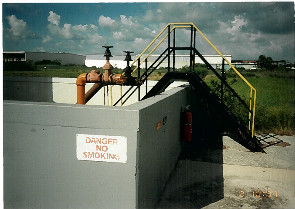
Photo 6d. The tanker truck hookup pipes and valves for waste solvents (brown pipe, to the right) and clean solvents (orange pipe, to the left). These pipes are used for transferring solvents to and from a tanker truck.
