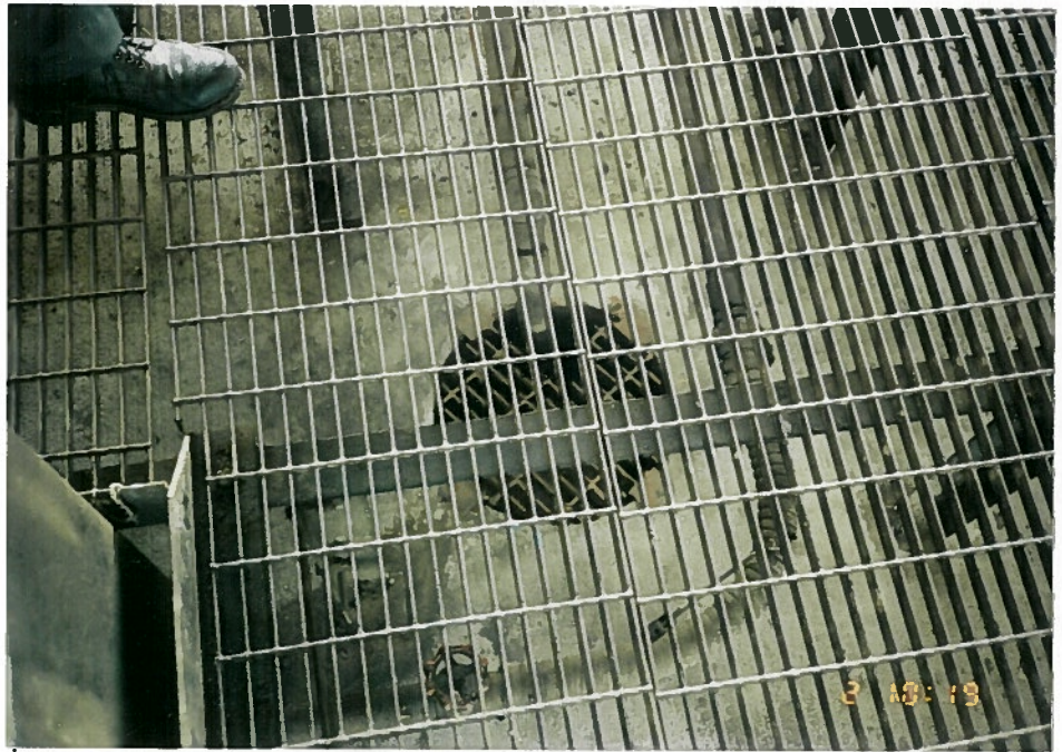
Photo 4a. Overview of the facility's solvent return fill shelters. The Solvent Return Wet Dumpsters (SWMU 3) are located here, and the Spill Containment Area Below the Fill Shelters (SWMU 4) can be seen beneath the metal grate platform.
