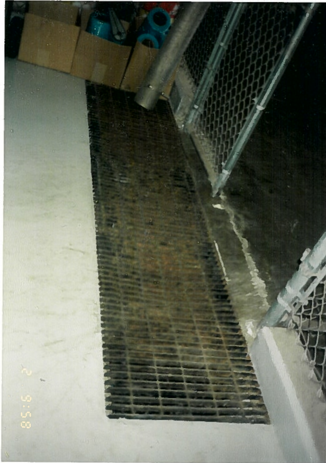
Photo 1b. Containment trench located in front of the Service Center Drum Storage Area (SWMU 1) gate.
