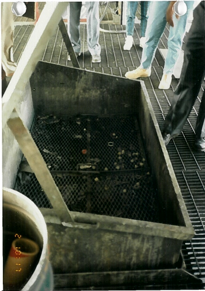
Photo 4b. This sump is located in the Spill Containment Area below the Fill Shelters (SWMU 4).
