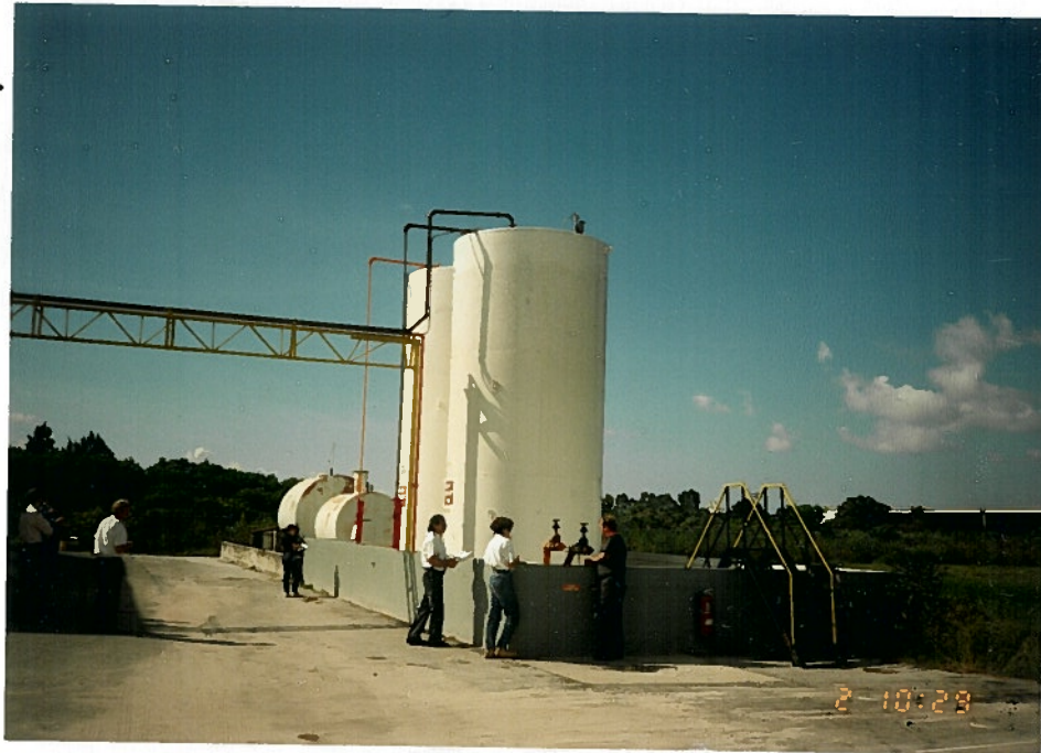
Photo 6a. Overview of the Waste Solvent Storage Tank area (SWMU 6), facing south. Note overhead piping to the tanks from the fill shelters.
