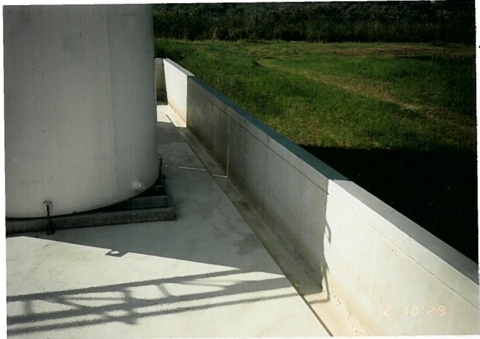
Photo 6c. Epoxy-coated concrete pad and cinder-block dike that surround the Waste Solvent Storage Tank area (SWMU 6). This view is facing south.
