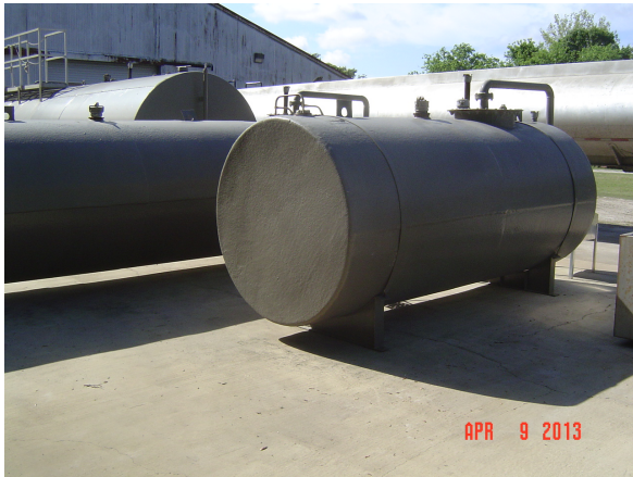
Photo 1 - used oil tanks
