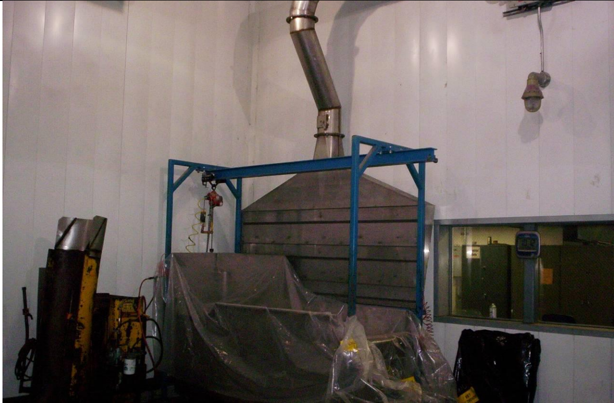
13. Debris Wash Unit
