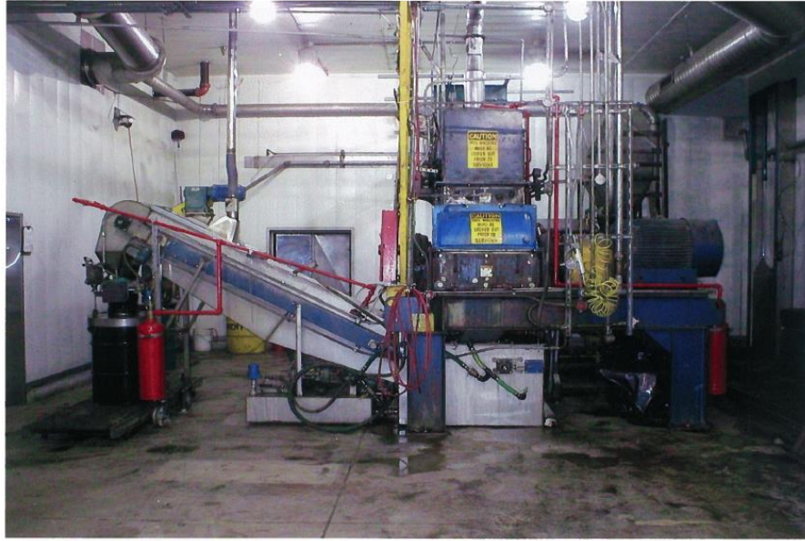
Figure 4. Image of LSV system as viewed looking north inside the LSV room.
