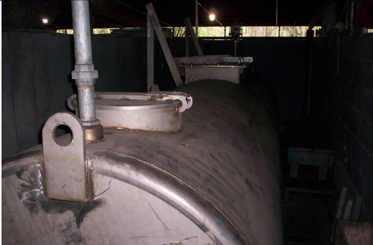
11. PSB 3,000-Gallon Storage Tank
