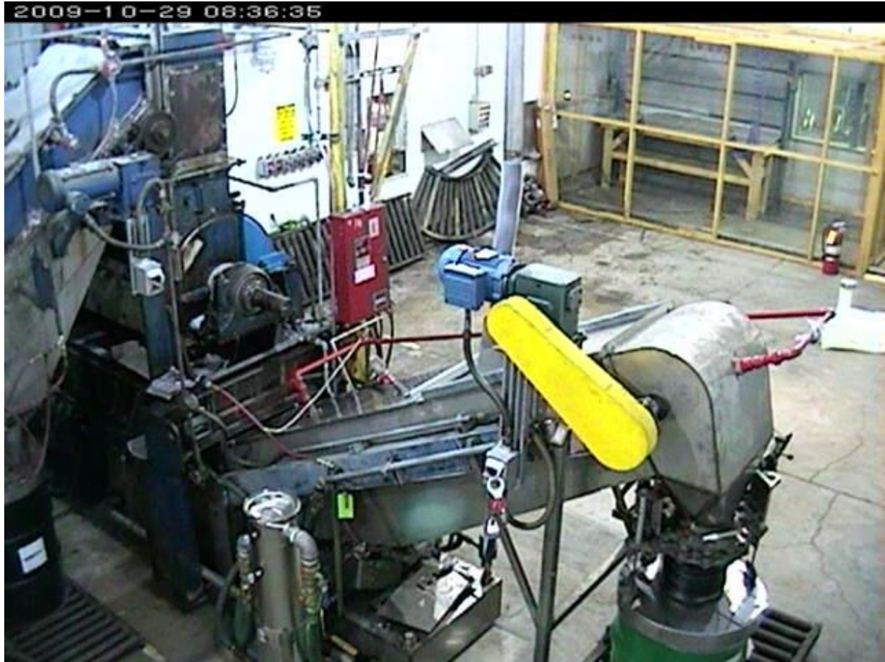
Figure I.D.10 LSV Process Equipment
