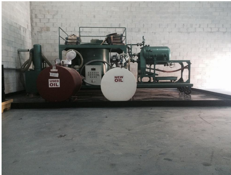
Description: View of Used Oil Processing/Regeneration Containment Area facing West. Note the concrete floor has been sealed with epoxy sealant
