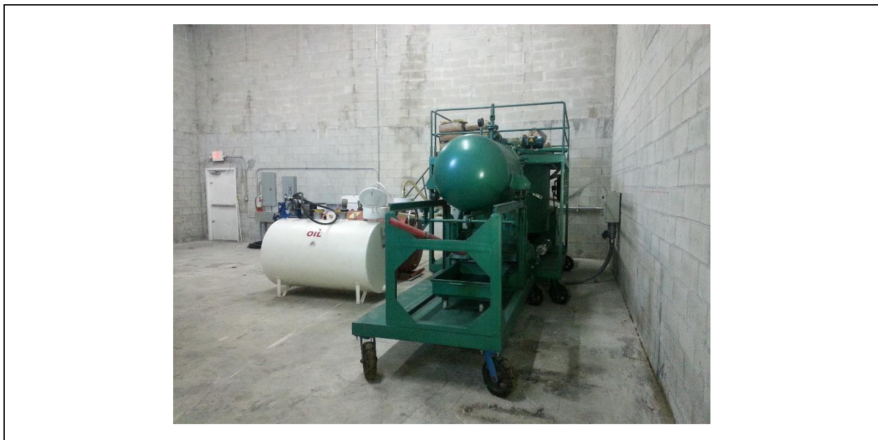
Description: View of the LYE-1000 Regeneration System showing Filter Press Tray for sludge collection facing South
