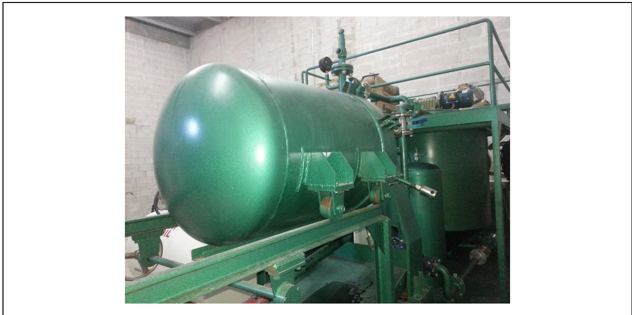
Description: View of the LYE-1000 Regeneration System & Vacuum Pump facing Southeast
