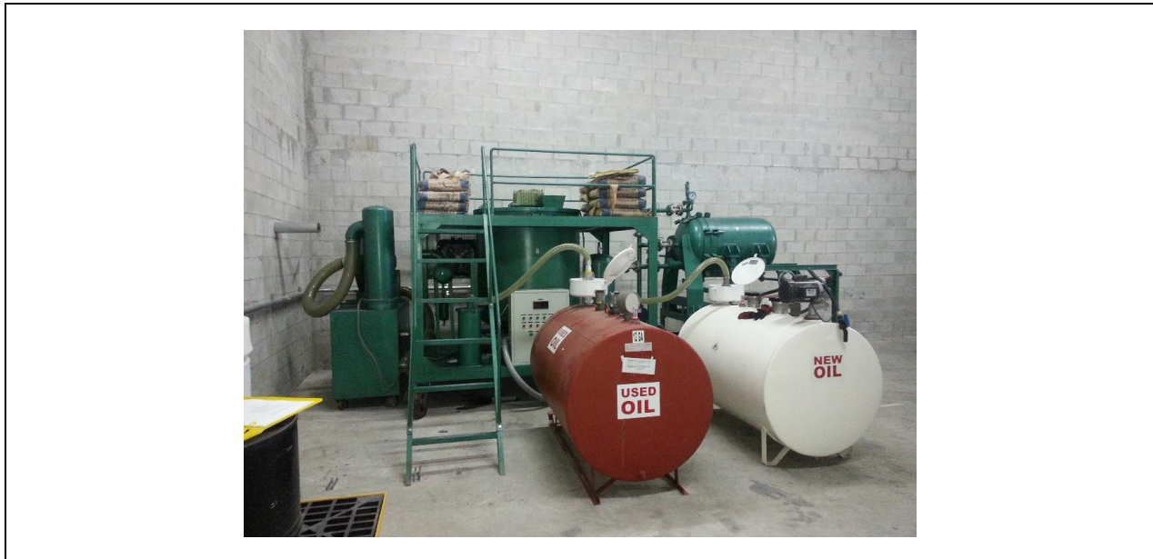
Description: View of the 295-gallon ASTs and the LYE-1000 Regeneration System facing West
