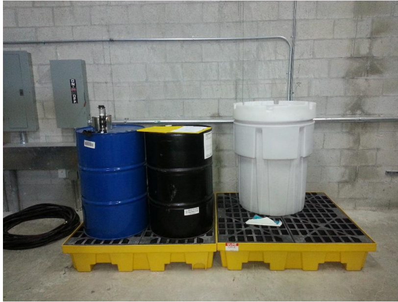
Description: View of New Chemical Storage & Waste Material Containment Area for 55-gallon Drums
