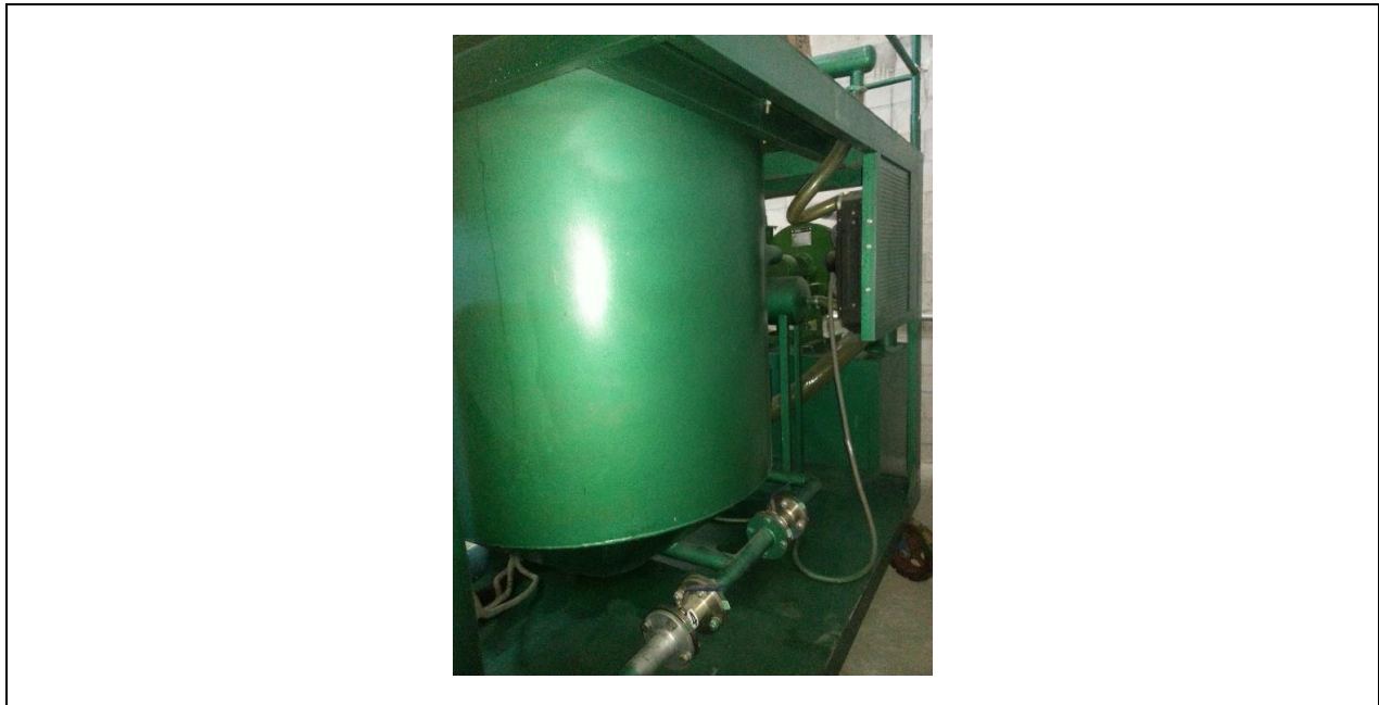
Description: View of the LYE-1000 Regeneration System & 300-gallon Reactor Tank facing Southeast
