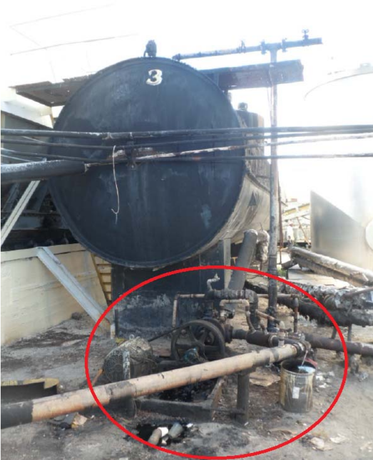
10. The photo below is taken at the paved pit area in front of the conveyor belt. There is pit approximately 2 x 5 ft sized filled with oily liquid inside. Please pump out the oily liquid and provide photos returned in compliance.
