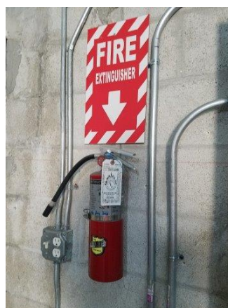
Fire extinguisher on site
