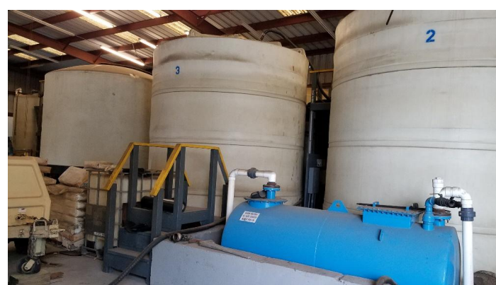
Wastewater Treatment Plant 1
