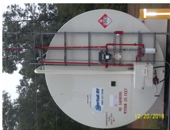
Photo 4 - Diesel Fuel Tank
