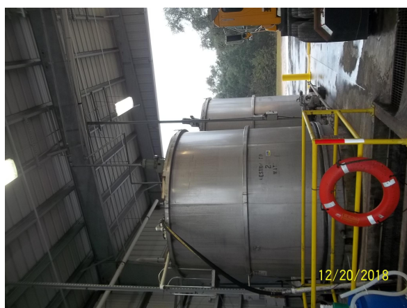
Photo 3 - Wash Rack Tanks
