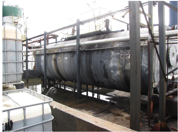
Used Oil/ Oily Water Treatment Tank
