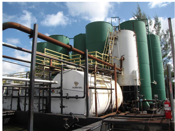
South Tank Farm
