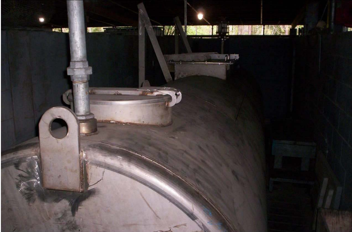
Photo 13. PSB 3,000-Gallon Storage Tank (12/2014)
