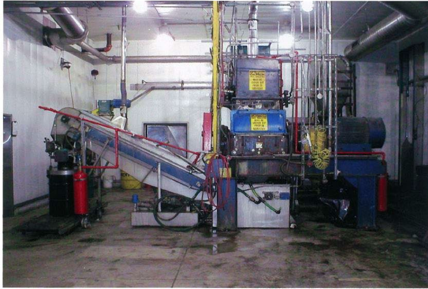
Figure 4. Image of LSV system as viewed looking north inside the LSV room.
