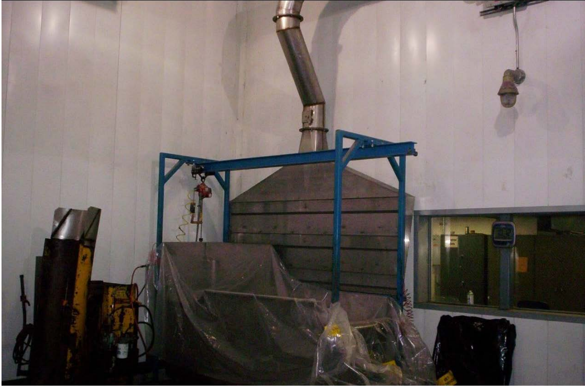
Photo 15. Debris Wash Unit (12/2014)
