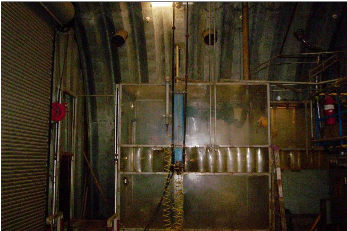
Photo 20. PF-I Treatment Room (12/2014)
