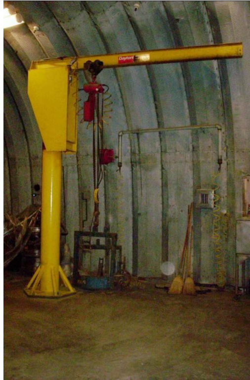
Photo 19. Quonset Hub Jib Crane (12/2014)
