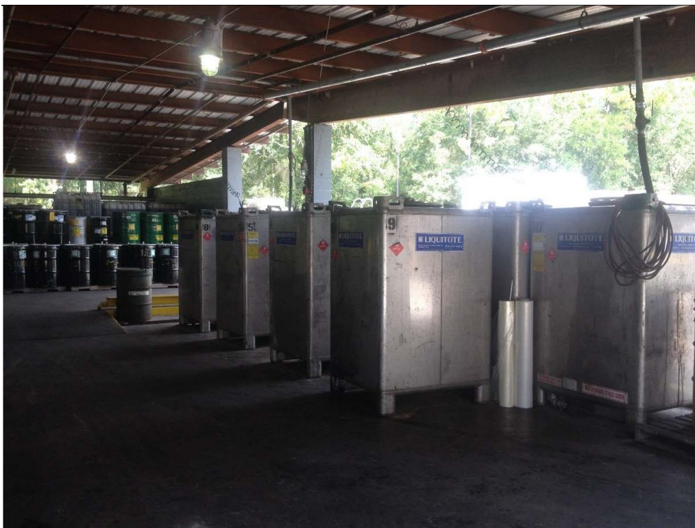
Photo 8. PSB Zone 1 Tanker Loading (12/2014)
