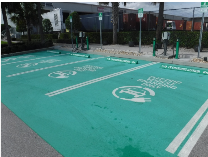
Electric Vehicle Charging Station (P2 Project)
