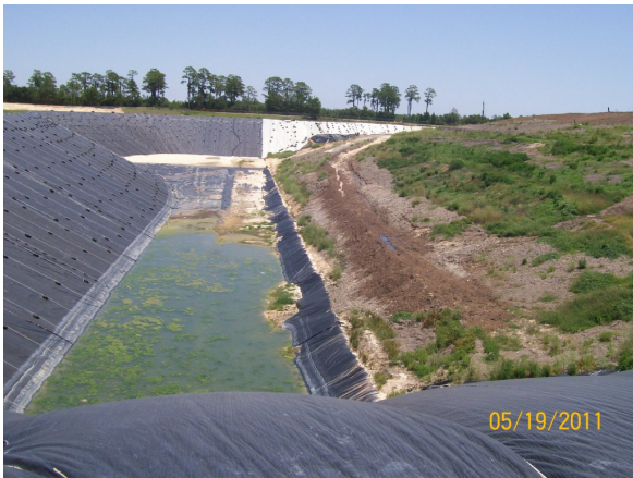
SW in Phase III, ponding@ N slope
