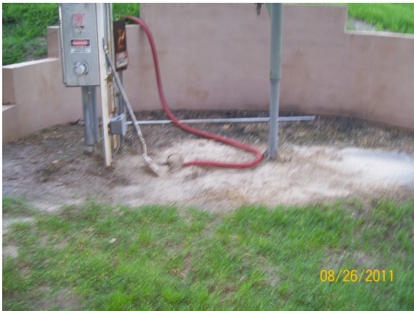
discharge to lift station
