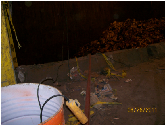
pump/hose in refuse pit
