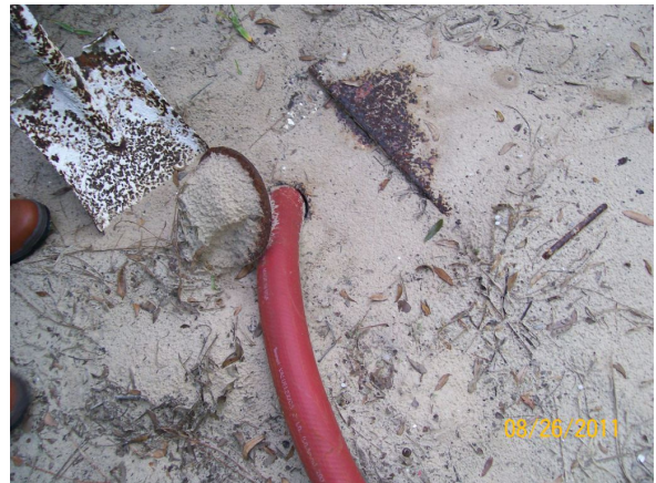
discharge to lift station
