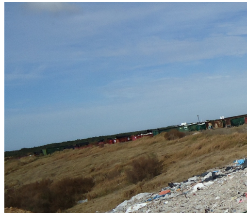
Newly Installed Gas Flares
