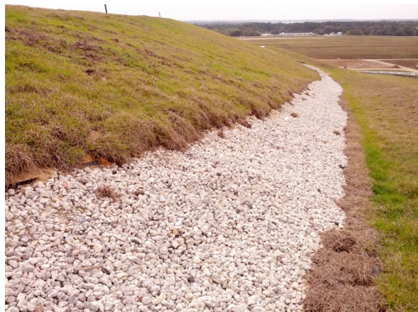
Deviated crushed concrete @ toe
