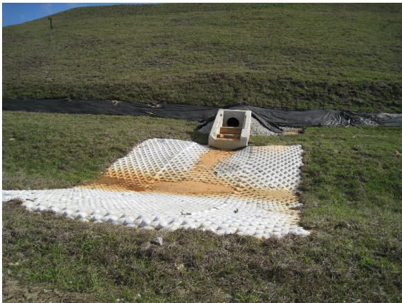
Stormwater Exit Pipe
