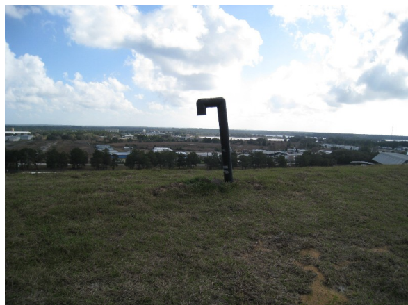
Passive gas vent
