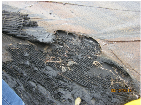
damage to geocomposite
