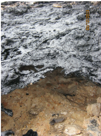
liner damage to subgrade, erosion
