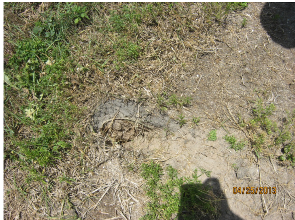
SW-1 broken off stand pipe
