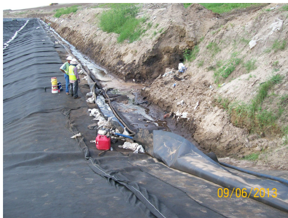
Leachate Issue at Intercell Berm
