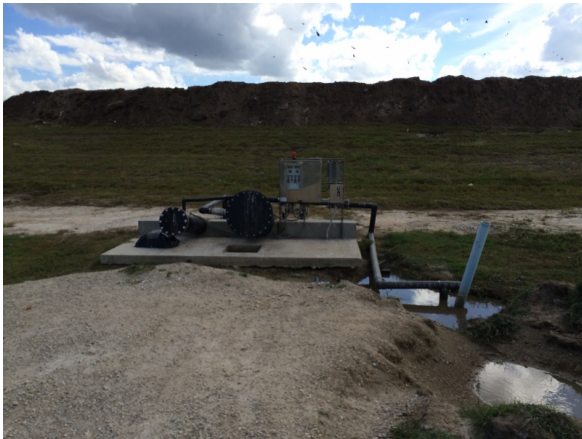
Leachate Spill Area
