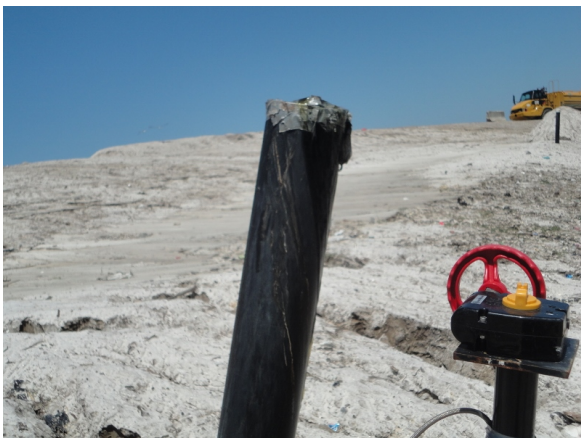
Well head Leachate Flow
