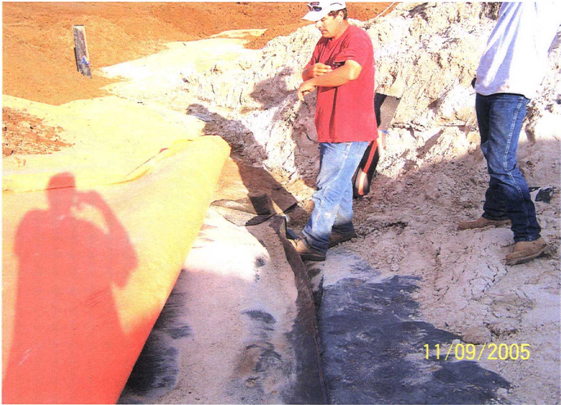
Attachment 2 – Photograph of “Blow-out” of separation berm. No damage to geomembrane
