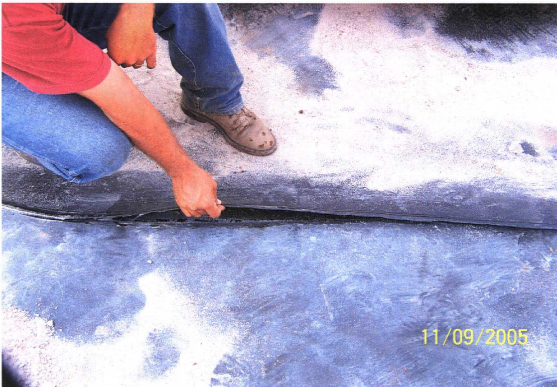
Attachment 2 – Close-up of “Blow-out” along separation berm extrusion weld
