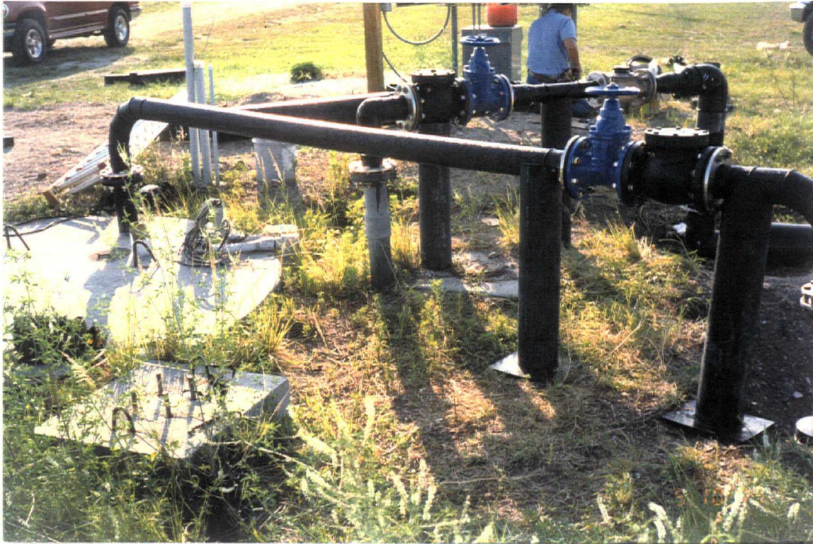
Date: May 10, 1999 Site: Southeast County Landfill, Hillsborough County, FL Description: PPS-A completed piping system (looking northeast).
