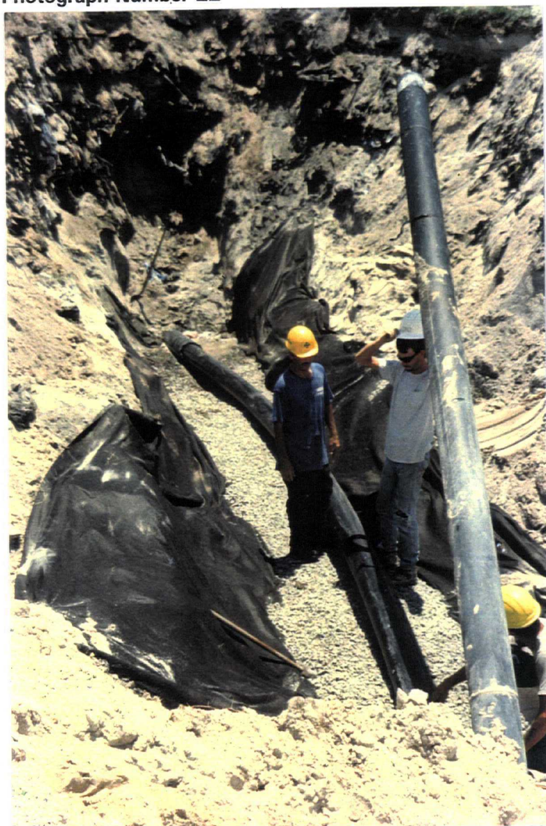
Date: May 20, 1999 Site: Southeast County Landfill, Hillsborough County, FL Description: Adjusting pipe length for tie in to Phase VI internal berm gravel Trench No. 3 (looking east).
