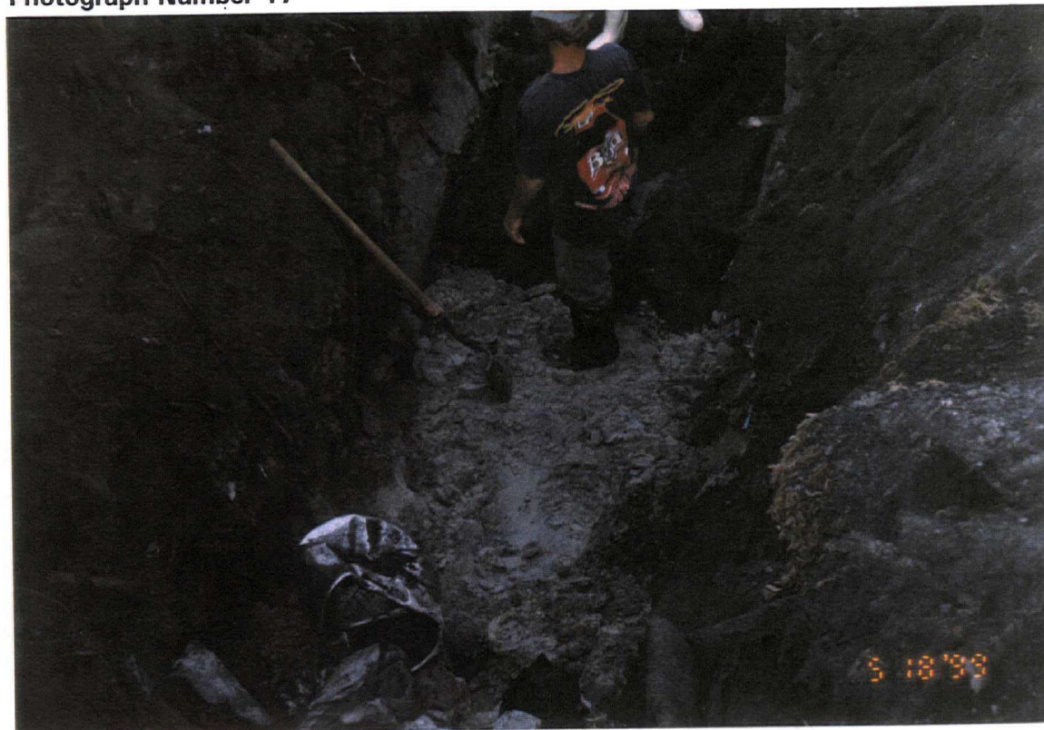
Date: May 19, 1999 Site: Southeast County Landfill, Hillsborough County, FL Description: Phase III internal berm chipped tire Trench No. 10 (looking west).
