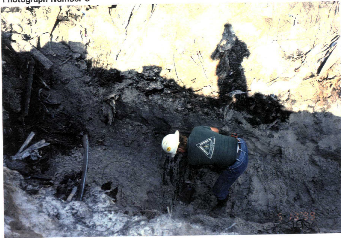
Date: May 13, 1999 Site: Southeast County Landfill, Hillsborough County, FL Description: Phase IV internal berm chipped tire Trench No.14 (looking west).
