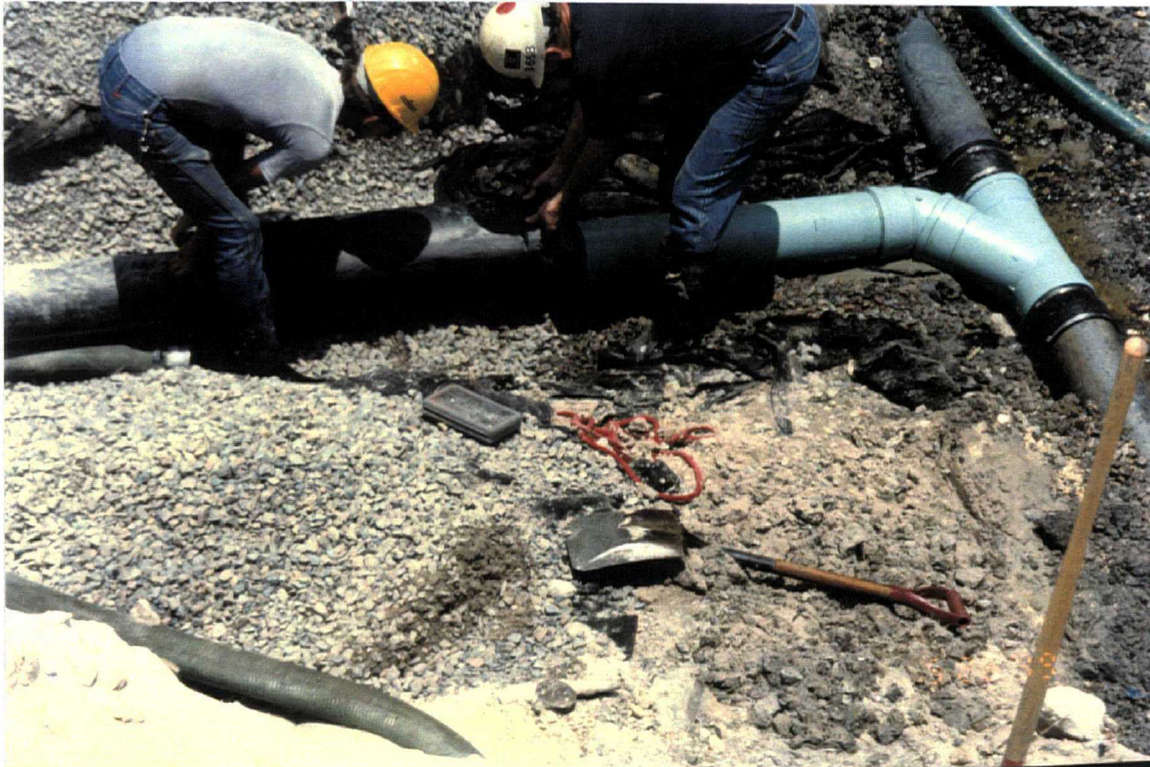
Date: May 25, 1999 Site: Southeast County Landfill, Hillsborough County, FL Description: Phase IV internal berm gravel Trench No. 4 (looking east).
