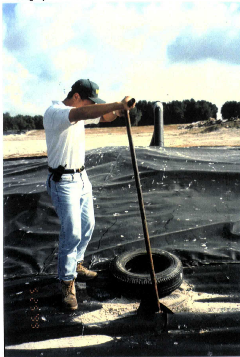
Date: May 25, 1999 Site: Southeast County Landfill Hillsborough County, FL Description: Opening valve No. 2 (looking north).
