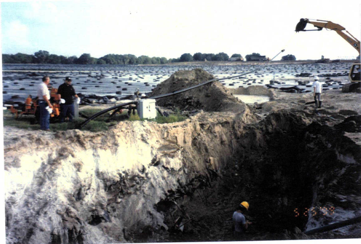
Date: May 25, 1999 Site: Southeast County Landfill, Hillsborough County, FL Description: Removal of TPS-5 suction line (looking northwest).
