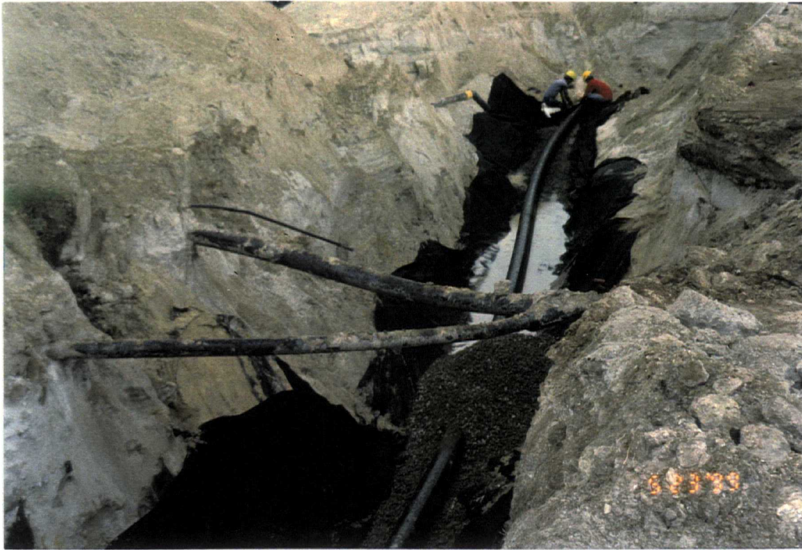
Date: May 22, 1999 Site: Southeast County Landfill, Hillsborough County, FL Description: Phase VI internal berm gravel Trench No. 4 (looking northwest).
