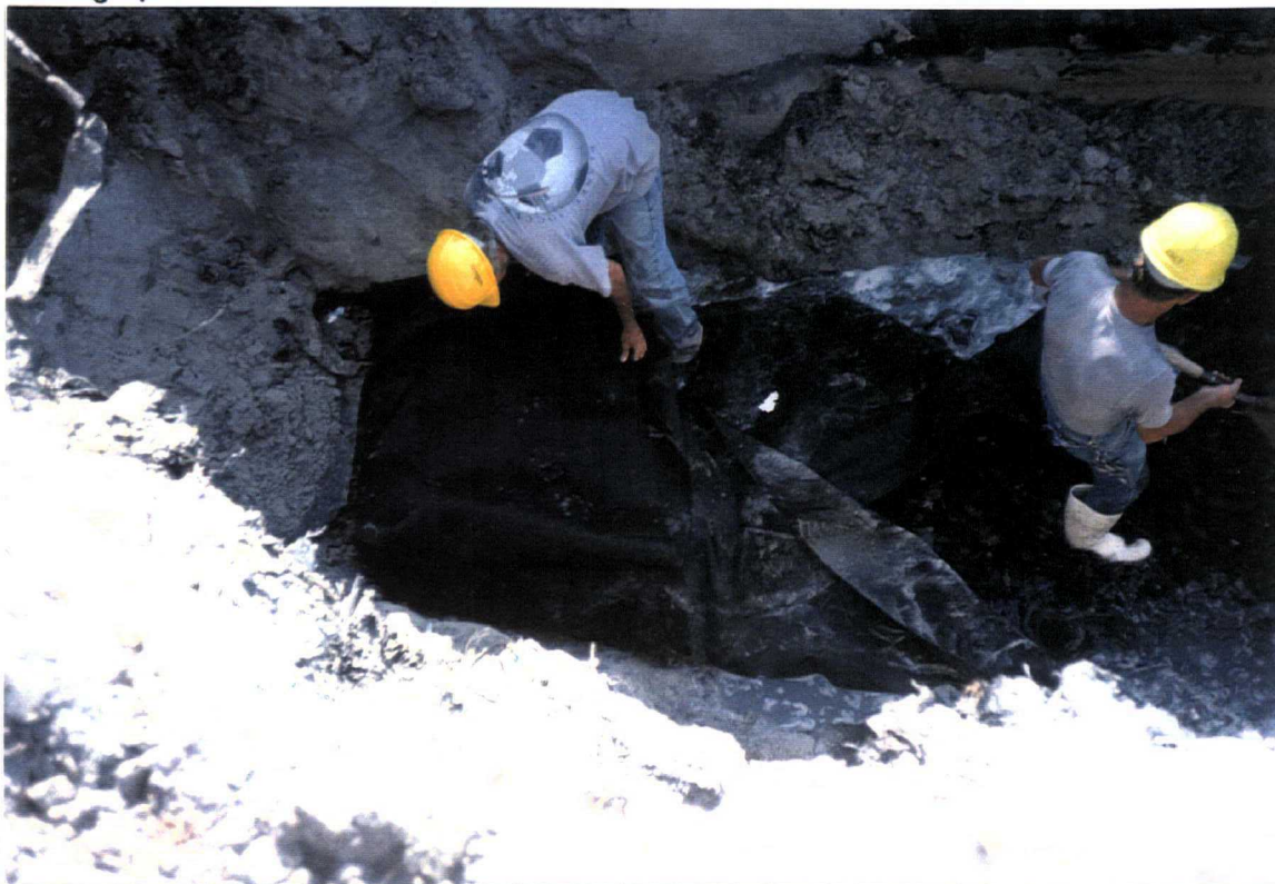
Date: May 17, 1999 Site: Southeast County Landfill, Hillsborough County, FL Description: Phase IV internal berm chipped tire Trench No. 12.
