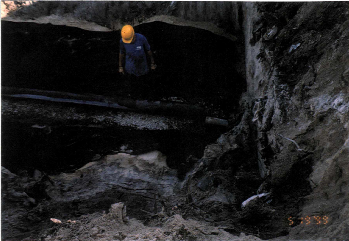
Date: May 20, 1999 Site: Southeast County Landfill, Hillsborough County, FL Description: Phase III internal berm gravel Trench No. 2 (looking north).
