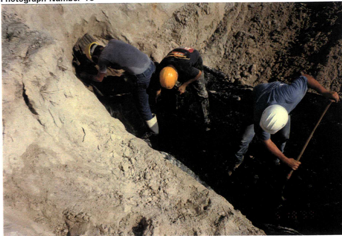
Date: May 19, 1999 Site: Southeast County Landfill, Hillsborough County, FL Description: Phase VI internal berm chipped tire Trench No. 10 (looking north).
