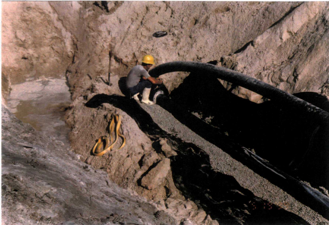
Date: May 20, 1999 Site: Southeast County Landfill, Hillsborough County, FL Description: Phase VI internal berm gravel Trench No. 2 (looking northwest).
