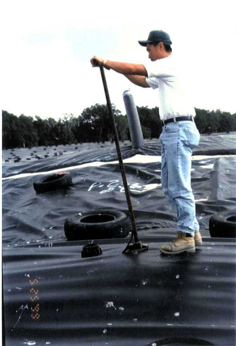
Date: May 25, 1999 Site: Southeast County Landfill Hillsborough County, FL Description: Opening valve No. 1 (looking north).
