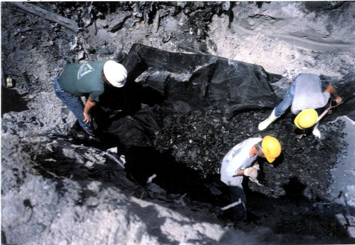
Date: May 17, 1999 Site: Southeast County Landfill, Hillsborough County, FL Description: Phase IV internal berm chipped tire Trench No. 13 (looking southwest).
