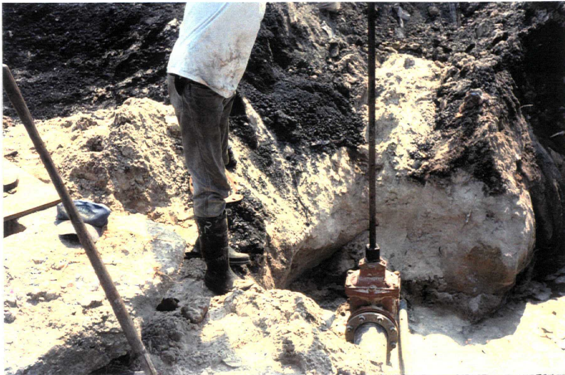
Date: May 11, 1999 Site: Southeast County Landfill, Hillsborough County, FL Description: Opening Valve Number 6 (looking west).
