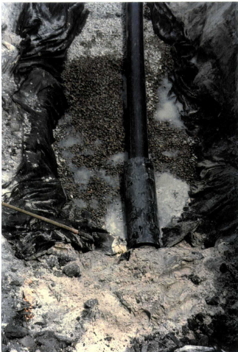
Date: May 21, 1999 Site: Southeast County Landfill Hillsborough County, FL Description: Phase IV internal berm gravel Trench No. 6 (looking north).
