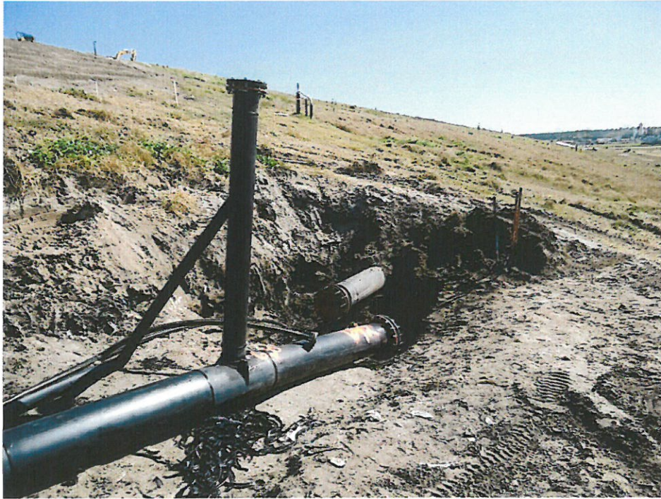
Point of Connection to Existing Header with Access Point
