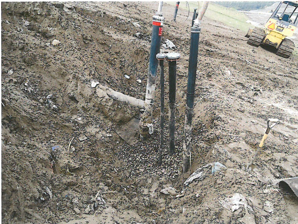
4" Condensate Force Main & 2" Compressed Air Line to Horizontal Collector
