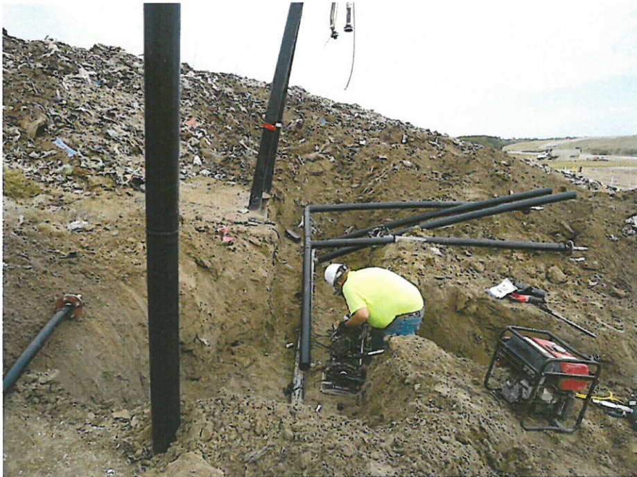
Installing new Air and Force Main for Horizontal Collectors on South Slope
