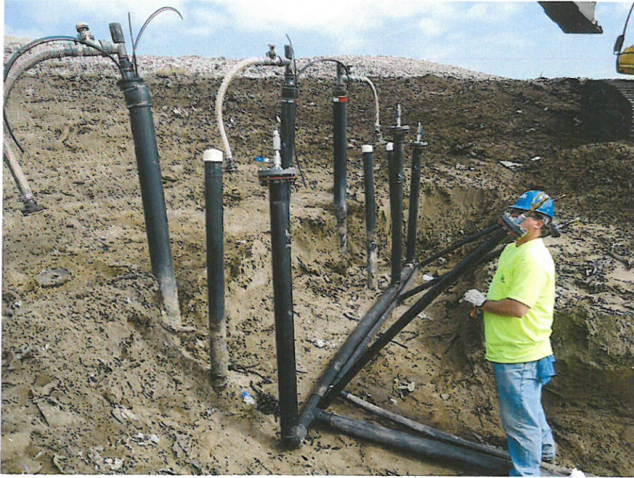
Installing new Air and Force Main for Horizontal Collectors on South Slope
