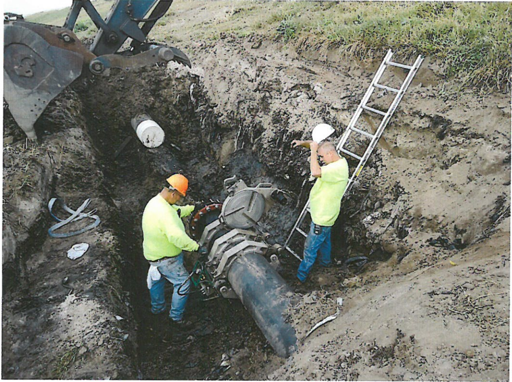
West Slope Header Point of Connection
