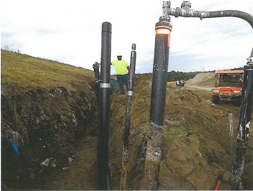
4" Condensate Force Main & 2" Compressed Air Line to EW-68
