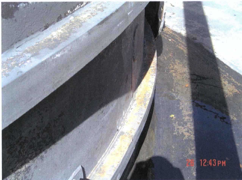
11. Stiffner corrosion in aeration section.
