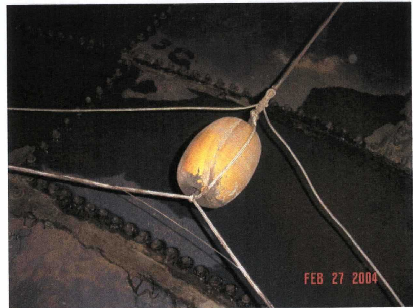
16. Cathodic protection float
