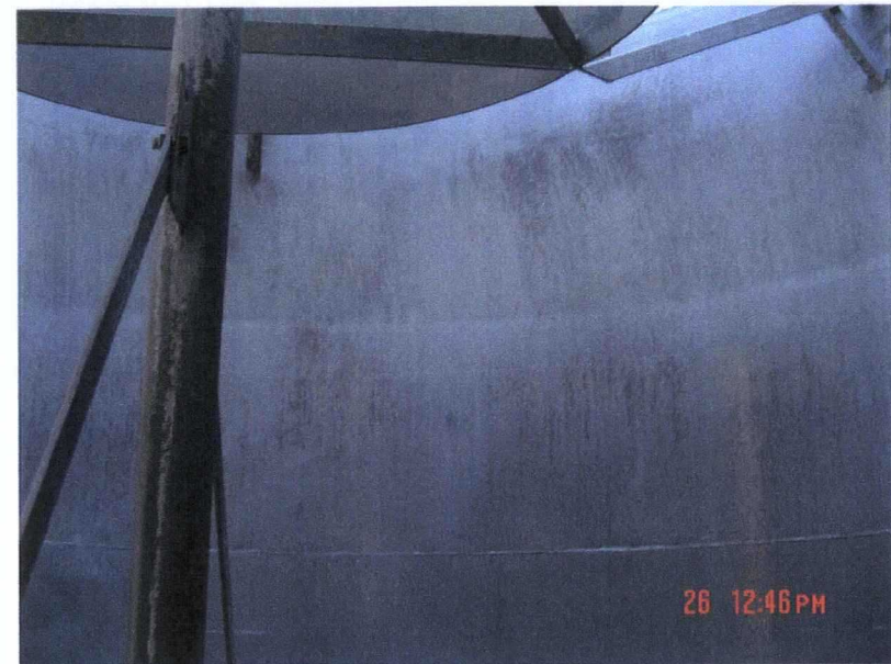
14. Clarifier center top.
