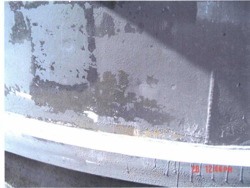
12. Wall corrosion in aeration section.
