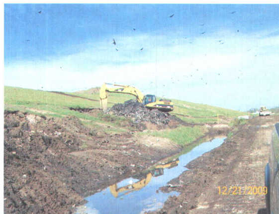
Leachate Seeps Being Repaired
