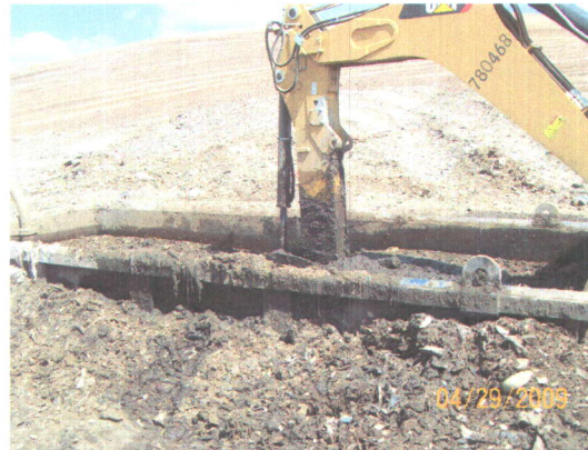
Waste Solidification Area
