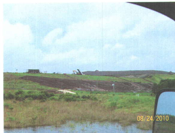
East Side Erosion
