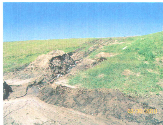
East Side Erosion
