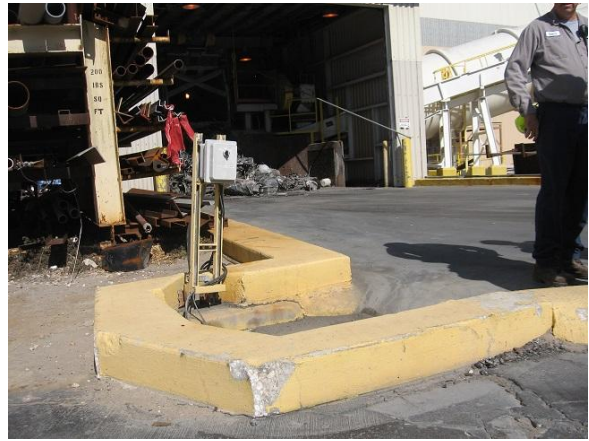
WTE Grizzly Leachate Sump/Pump
