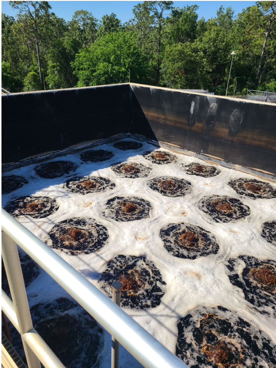
Photo 4: South Leachate Tank filled, and all diffusers are working designed.
