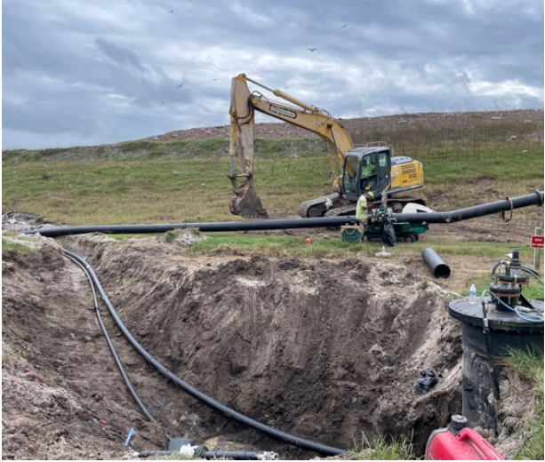
12-inch Header Connection to CS-9
