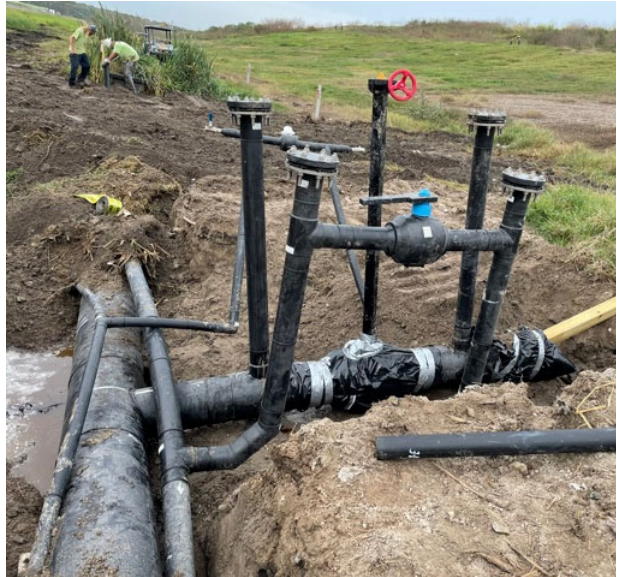
16-inch Header Line Connection to CS-13
