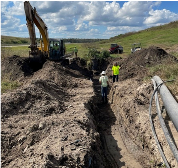
16-inch Header Connection to CS-13
