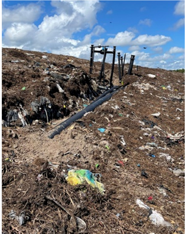
Valve Pit and Access Point in Header
