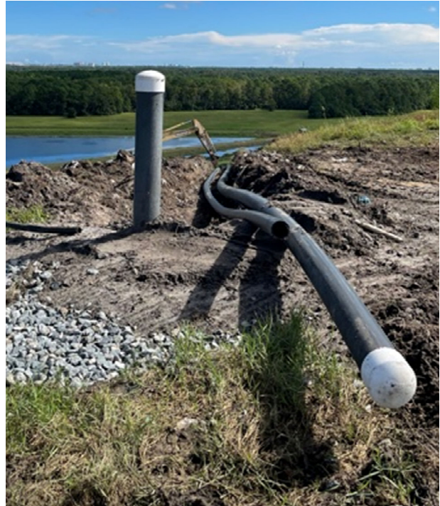
Vertical Well, Forcemain and Air Line
