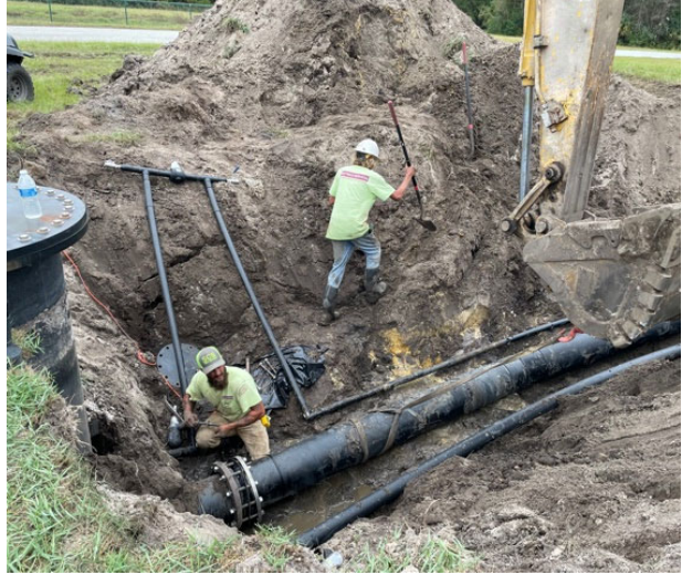
12-inch Header Connection to CS-9
