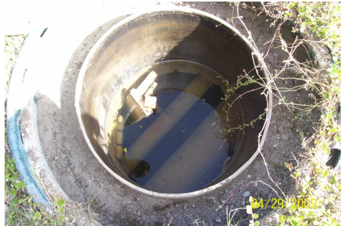
db wall leachate pipe containment
