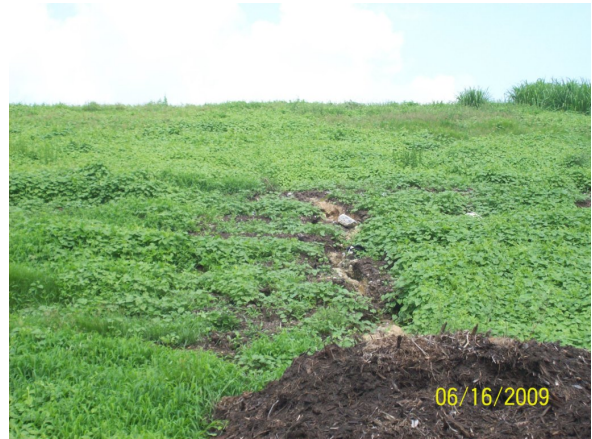
Erosion on east slope.
