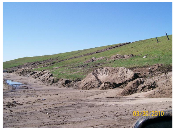
East Side Erosion
