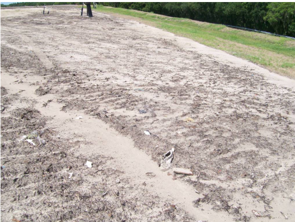
Phase V - erosion w/exposed waste
