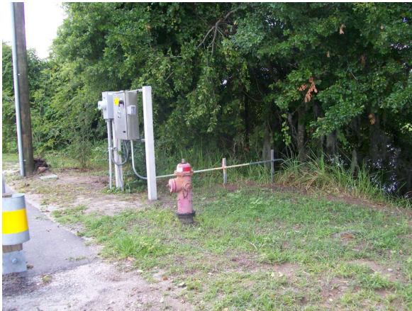
new fire hydrant
