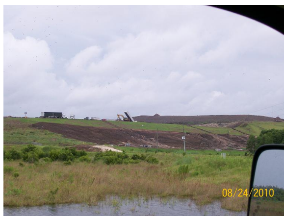
East Side Erosion
