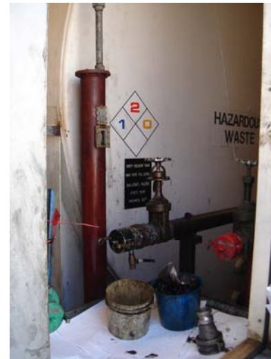
Tank Load/Unload valves
