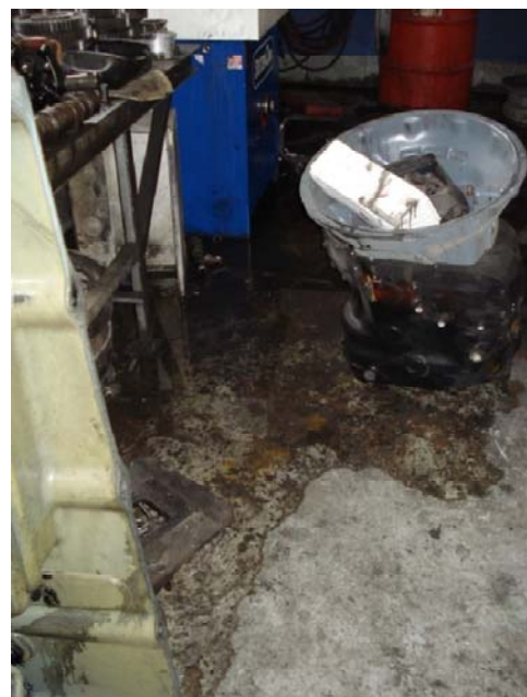
Figure 6: Water intrusion from leaking roof
