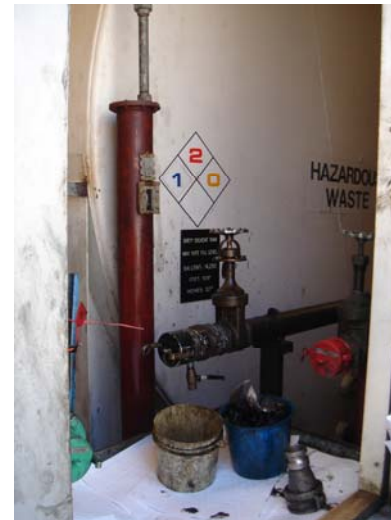
Tank Load/Unload valves
