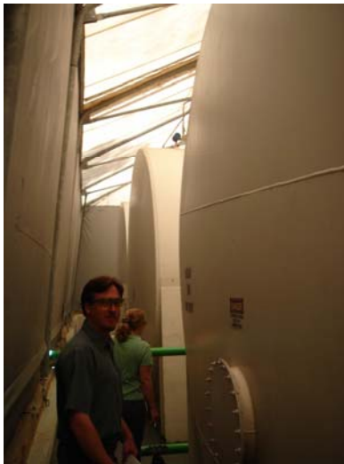
East end of Tank Farm
