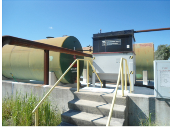
New separator & Used oil tank
