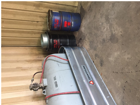
Photo 1 - RTC Used Oil Secondary Containment
