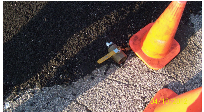
Secondary containment drain valve
