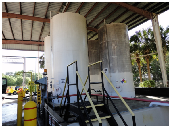
Fig 6: Above Ground Storage Tanks
