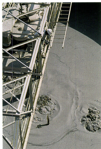
Slurry is held in correcting tanks for adjustments in composition.
