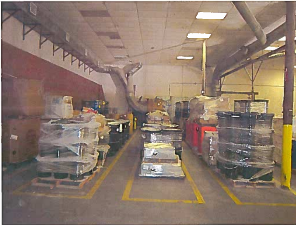
Photograph 5 – Bulb and battery staging area.
