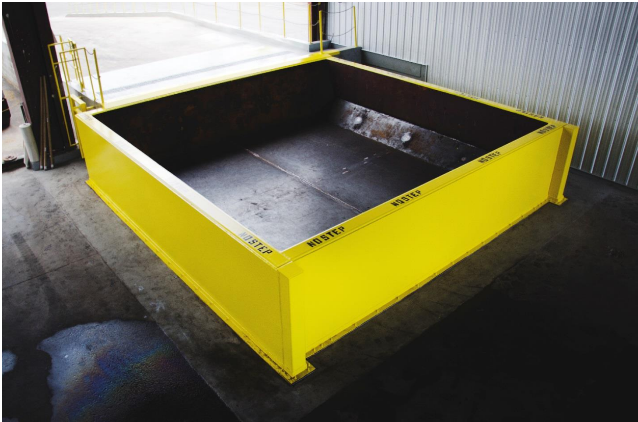
SWMU 7 – Waste Processing Building - Hazardous Waste Treatment Tank. This photograph shows the hazardous waste treatment tank, facing south west. Photo taken 2014.
