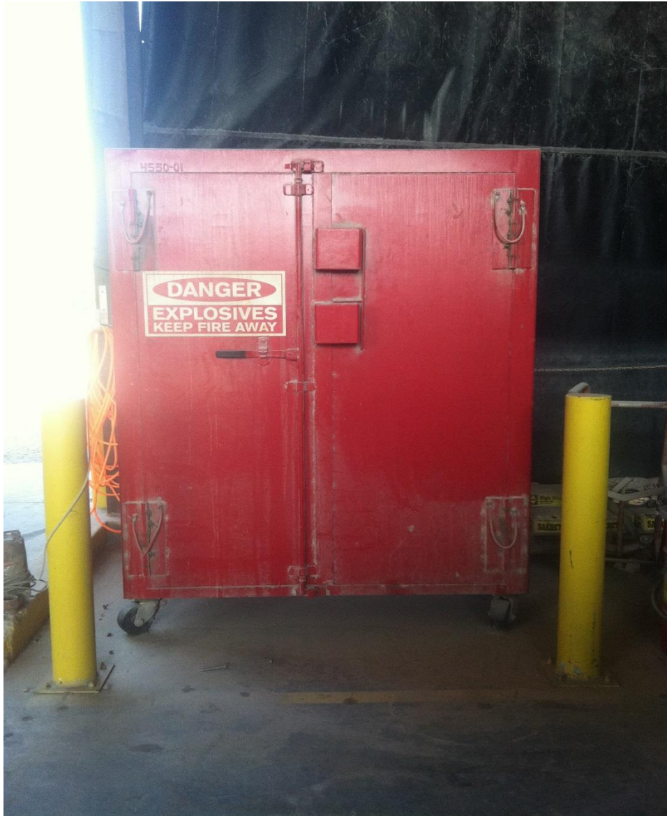
SWMU 7 – Waste Processing Building – Reactives Magazine. This photograph shows the reactives Magazine hazardous waste treatment tank, facing west. Photo taken 2016.
