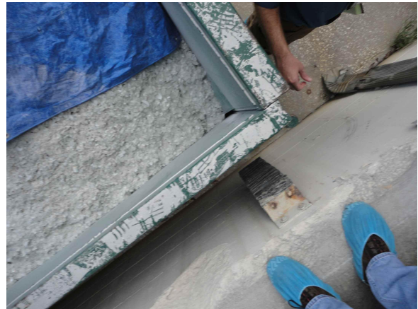
14. Processed glass container gate - not sealed
