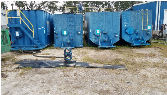
Empty Frac Tanks
