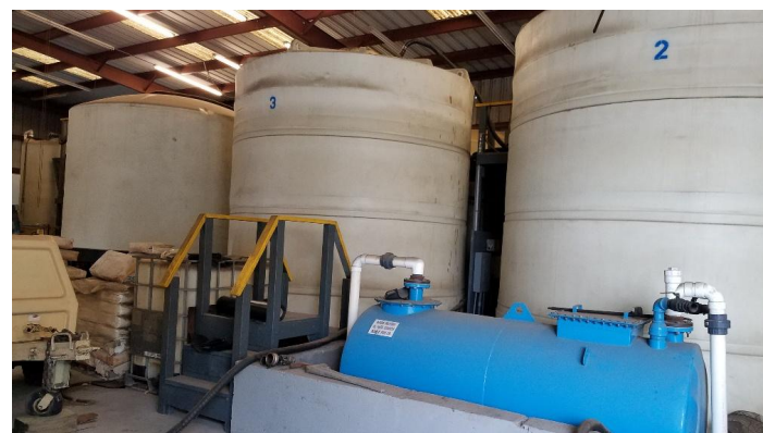
Wastewater Treatment Plant 1
