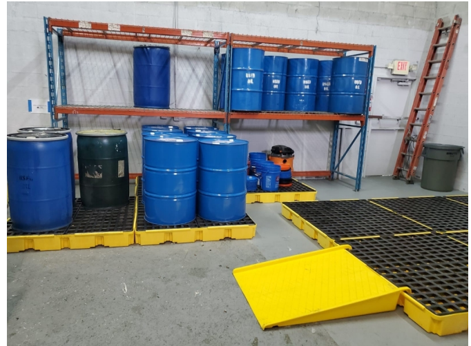
UO drums with secondary containment
