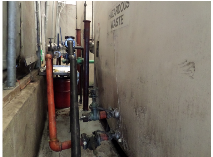
Photo 2: Hazardous Waste Tank & Lines
