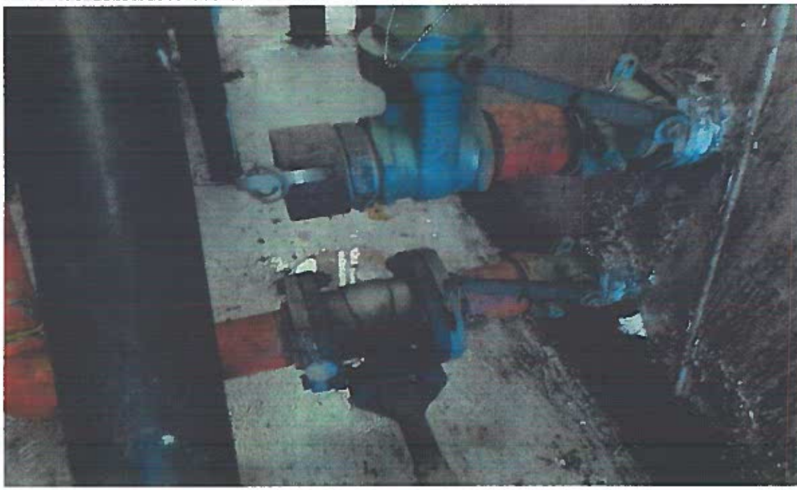
Safety Kleen Systems, Inc. – Tallahassee FL. RCRA Permitted Tank Farm. Inspectors observed one 15,000-gallon Tank marked with the words hazardous waste. Inspectors observed metal numbered tags on each valve, flange, and pipe connection. Photograph 3 taken at 12:22 p.m. WK.
