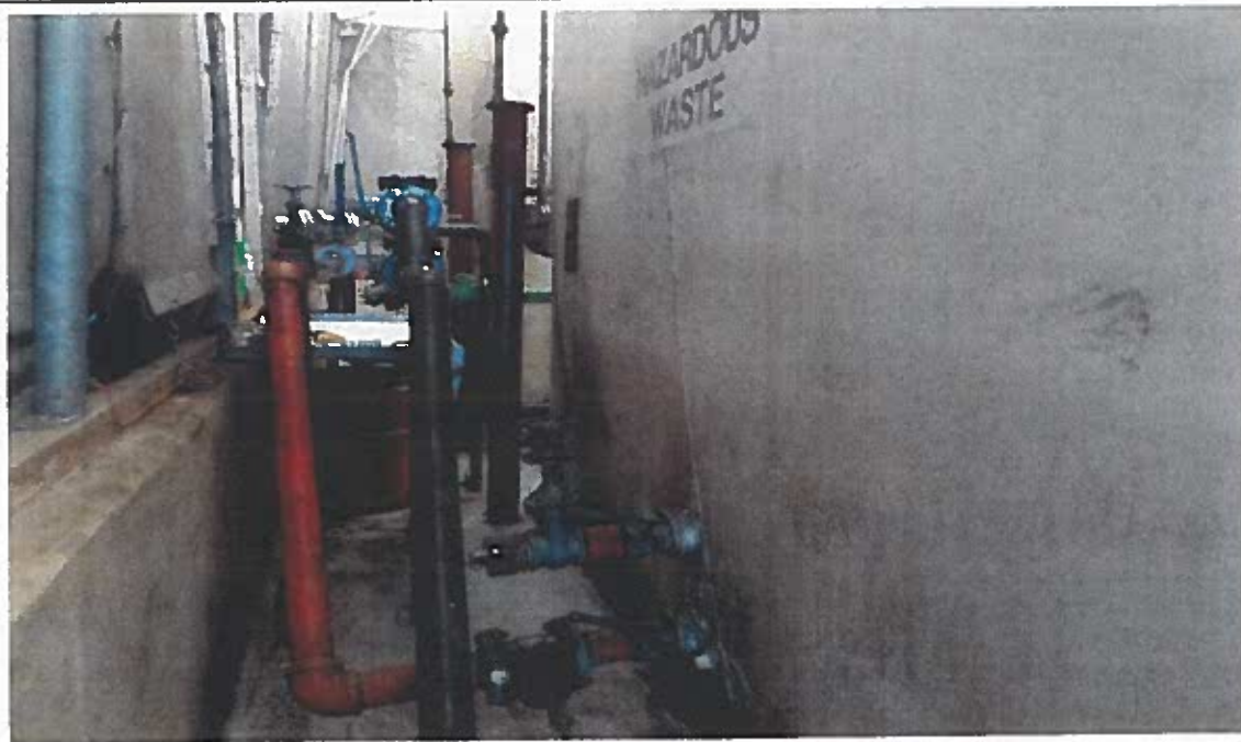
Safety Kleen Systems, Inc. – Tallahassee FL. RCRA Permitted Tank Farm. Inspectors observed one 15,000-gallon Tank marked with the words hazardous waste. Inspectors observed metal numbered tags on each valve, flange, and pipe connection. Photograph 2 taken at 12:22 p.m. WK.
