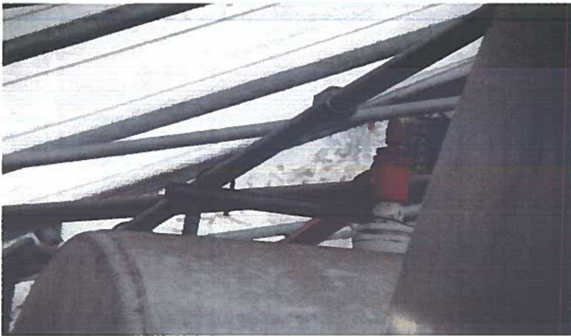
Safety Kleen Systems, Inc. – Tallahassee FL. RCRA Permitted Tank Farm. Inspectors observed one top mounted emergency vent and pressure/vacuum vent on the 15,000-gallon Tank. Photograph 4 taken at 12:22 p.m. WK.
